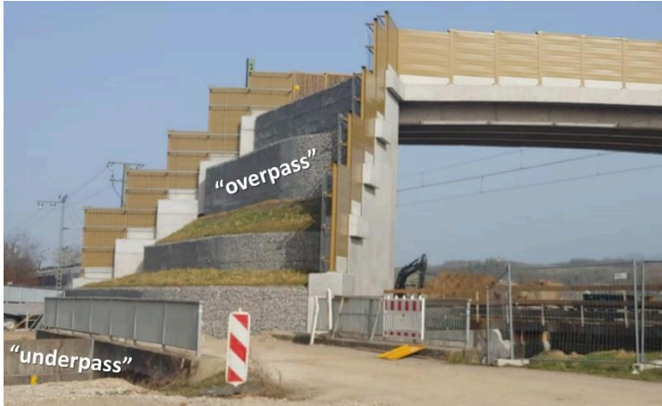
Figure 78: Recent construction site of inadequate fauna passages at an important corridor/watercourse in the Rhine valley
