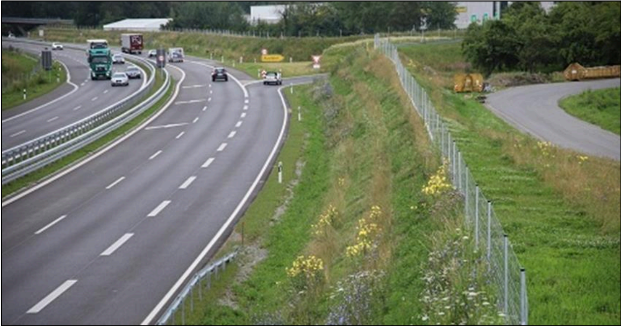
Figure 86: The minimum requirement for ecological functioning verges is the establishment of suitable maintenance regimes
